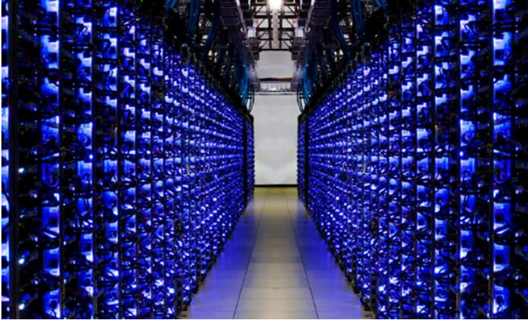
Data Center farm
